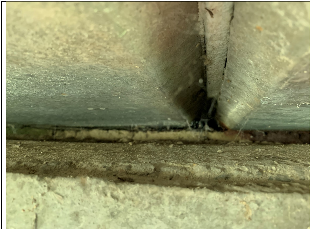
Photograph 3: Close up of crevices in northern and southern ends of bridge.
