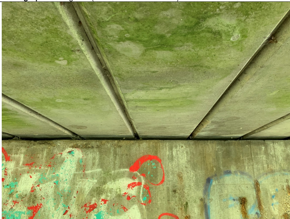
Photograph 2: Gaps in northern and southern ends of Bridge B8
