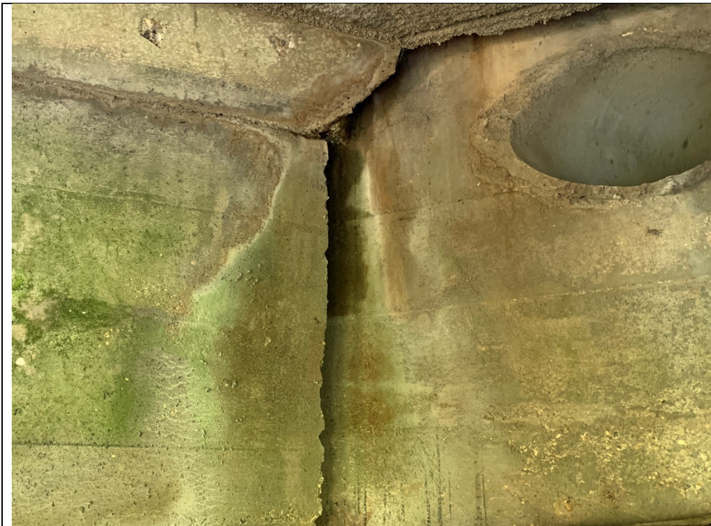
Photograph 7: Gaps behind concrete supports on northern and southern ends of Bridge B9.
