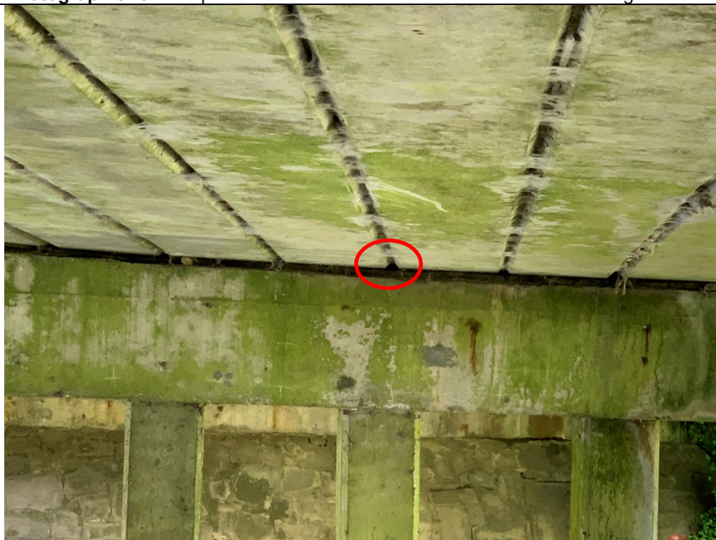
Photograph 4: Gaps in central supports of bridge B8
