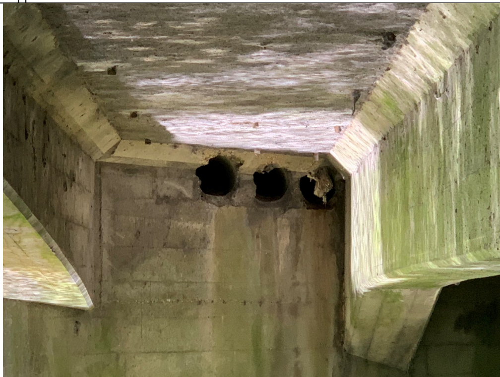
Photograph 6: Close up of pipe holes in central support
