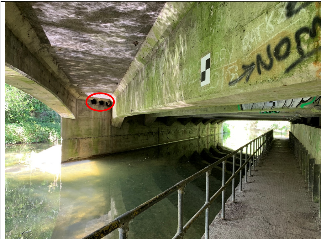
Photograph 5: Bridge B9 with more sealed structure and pipe holes into central supports.
